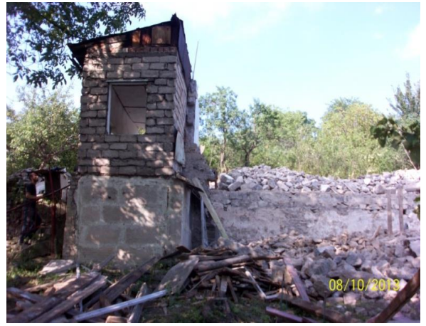
In August of 2013, the church was being demolished due to crumbling foundation.
